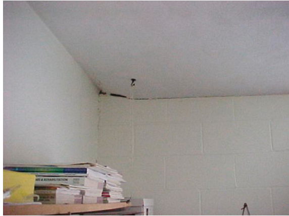
Fig. 27 Displacement of ceiling wall-board along non-load bearing walls due to floor heaving
