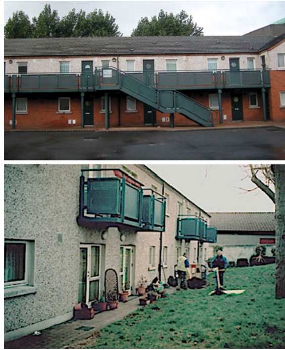
Fig. 3 Block 3, front elevation showing manholes and rear elevation showing location of trial pits
