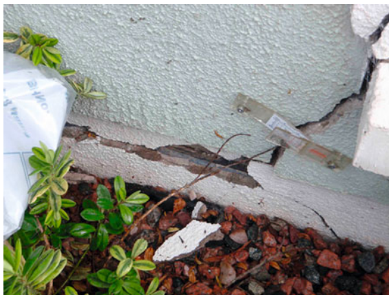
Fig. 1 Horizontal and vertical displacement due to pyritic heave in a domestic property in the Dublin area. The vertical displacement is of the order of 5–7 mm and the horizontal displacement is in excess of 10 mm
