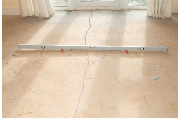
Fig. 9 Crack up to 7 mm wide across a floor which has risen 30 mm within a distance of 2.5 m
