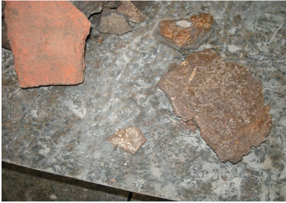
Fig. 15 Chunks of shale bedrock extracted from beneath floor slab
