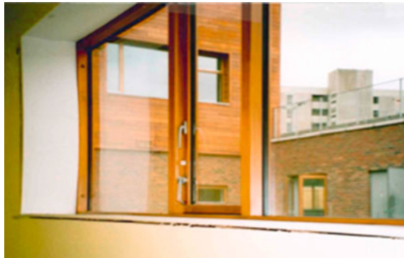
Fig. 15 Gap developing as window cill arches, between corridor from the Gym and the courtyard
