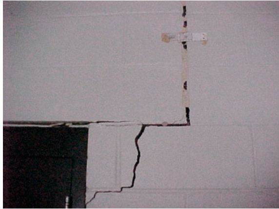
Fig. 25 Large cracks (1 inch) in concrete block adjacent to doorway. Note the attempt to bracket the wall cracks
