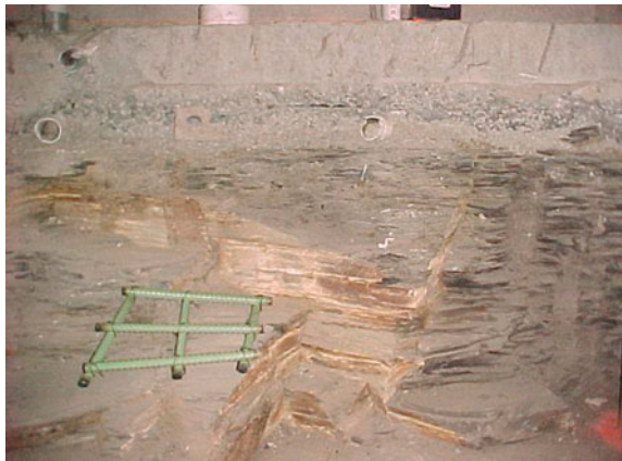
Fig. 17 Multidirectional cleat fractures with sulphate precipitates below walls. Note green re-bar
