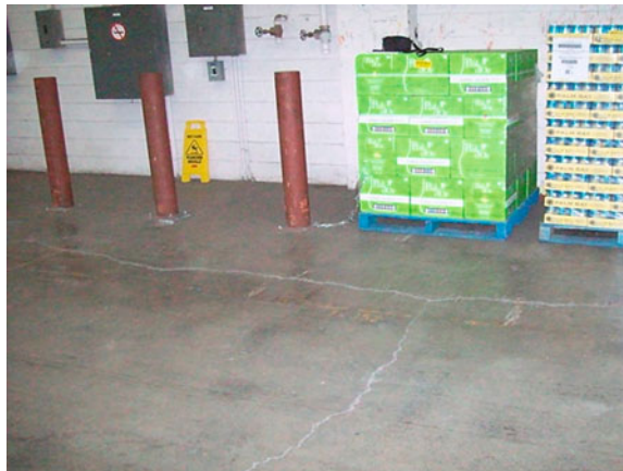
Fig. 12 Intersecting floor cracks indicative of upward heave of the slab
