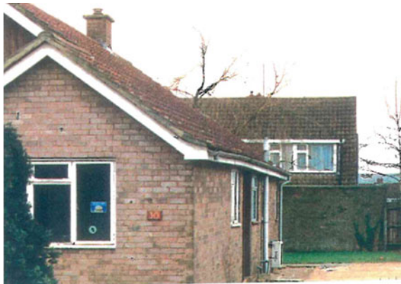
Fig. 51 Significant arch in front facade of the same bungalow as in Fig. 50
