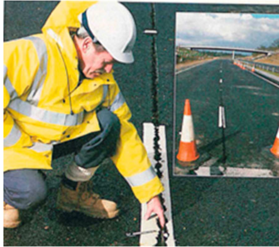
Fig. 55 Distress in the A10 (north of London) following lime stabilisation of sulphate-rich soils (New Civil Engineer 25 March 2004)
