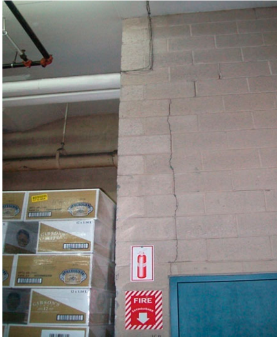
Fig. 13 Cracking in internal block wall supported on floor slab
