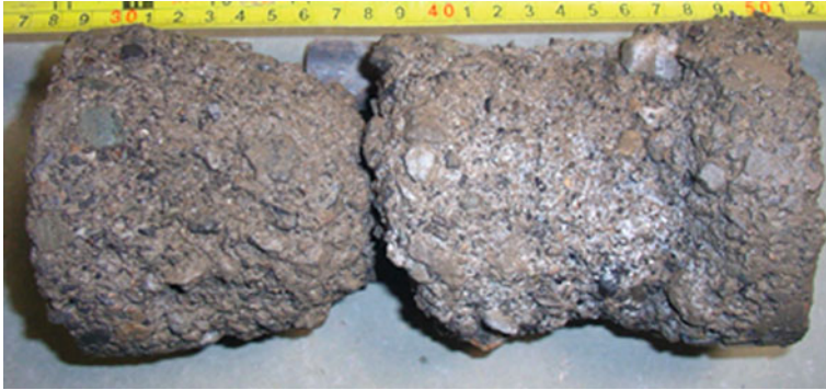
Fig. 61 Degraded concrete with thaumasite developed in poor quality block in a rising wall
