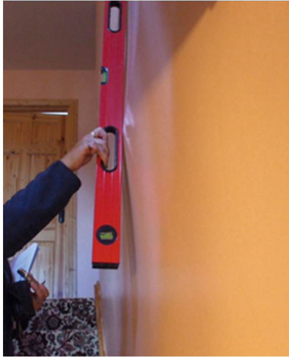
Fig. 11 Bowing of a stud wall pushed upwards by the rising floor slab
