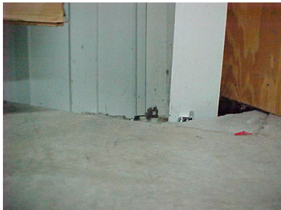
Fig. 24 Heaved floor adjacent to load-bearing wall on main floor of the Carhartt Factory. Note the cell phone resting on steel column for scale
