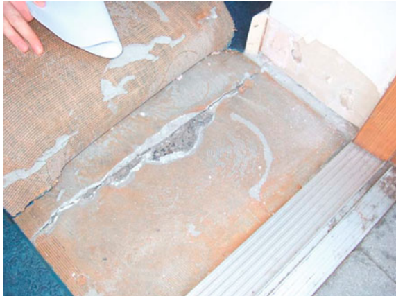
Fig. 17 Rise of floor against the threshold into the stairwell (November 2007)
