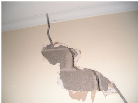
Fig. 10 Cracking through plaster and blockwork of internal wall
