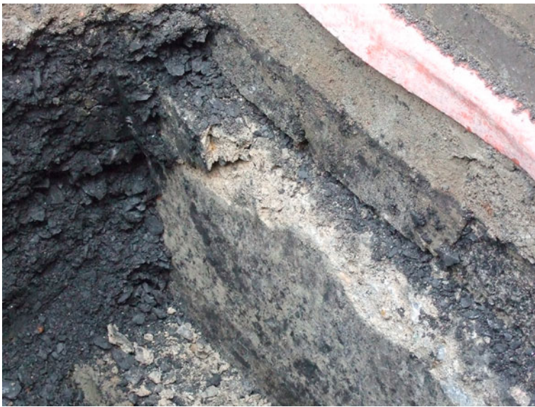
Fig. 28 Deterioration of concrete at the top of the beam, TP 11, and the nature of the dark deleterious fill adjacent to it
