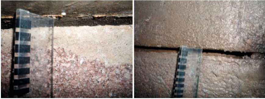
Fig. 73 Rise of a manhole biscuit/cover slab of up to 13 mm due to the expansion of the surrounding pyritiferous fill ( left ). In the manhole wall itself gaps of up to 10 mm were noted ( right ) where the upper wall remained cemented to the biscuit
