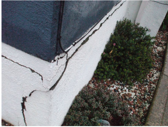
Fig. 5 Cracks created during lateral displacement of a rising wall
