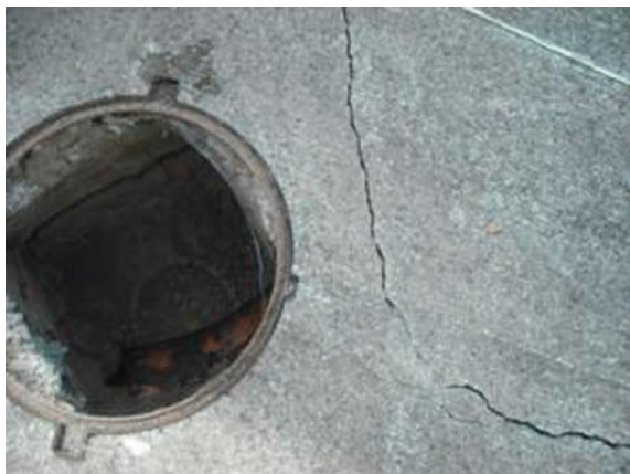
Fig. 21 Pavement cracking near manhole
