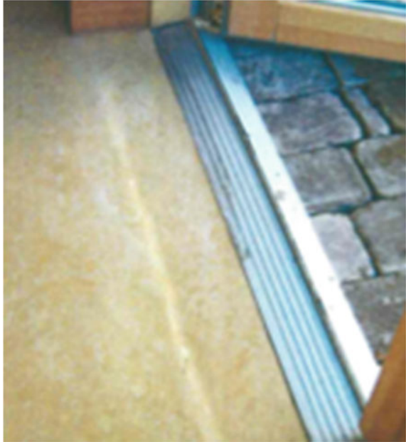
Fig. 16 Damage to threshold at doorway from Reception into the courtyard (March 2007)
