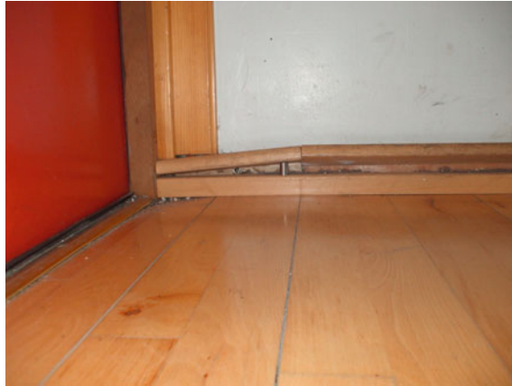
Fig. 12 Displacement of timber skirting
