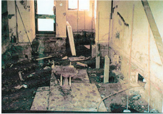
Fig. 49 Remediation included installation of piles to support suspended floor slabs at Hucclecote
