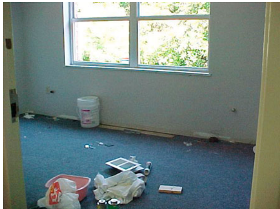
Fig. 28 Repair of floor, walls and copper water lines damaged by office floor heave
